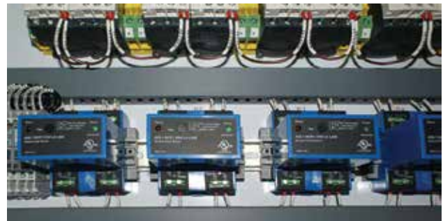
A typical installation of ground fault sensors monitoring several heating circuits used in the semiconductor fabrication process. If a fault to earth is detected, the latching output sensor de-energizes the contactor coil, turning off the offending circuit.
