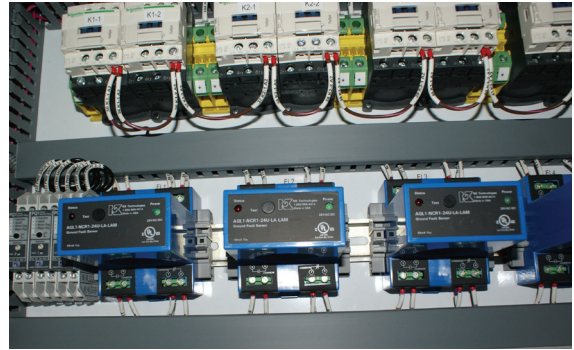
A typical installation of ground fault sensors monitoring several heating circuits used in the semiconductor fabrication process. If a fault to earth is detected, the latching output sensor de-energizes the contactor coil, turning off the offending circuit.
