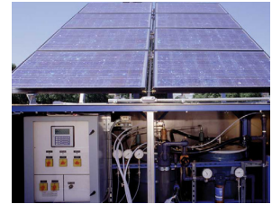
Monitor solar panels to ensure they are producing the correct amount of DC voltage.
